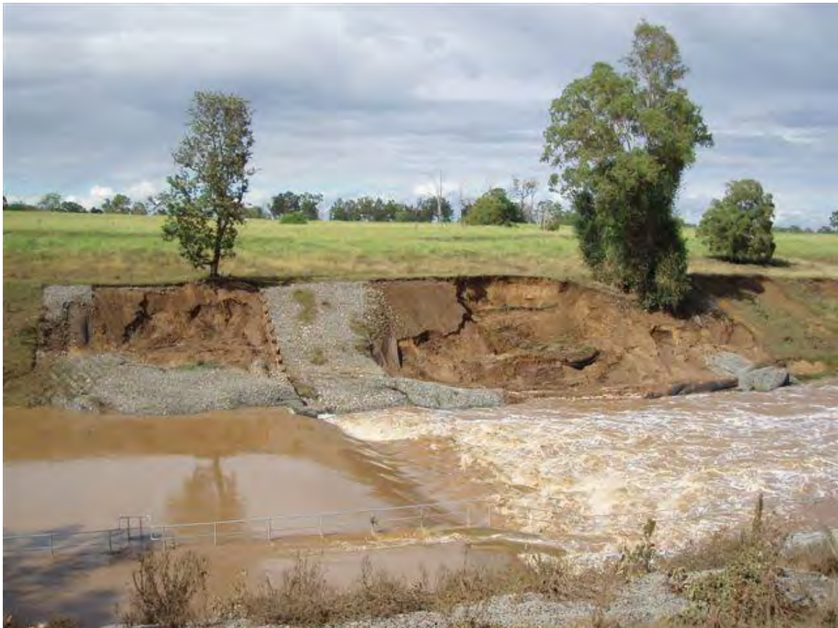
Figure 24 South Maclean Weir – Logan River - Slumping of bank protection works
